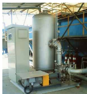
30-kW micro-bubble aerator (Shanghai's textile factory C)
