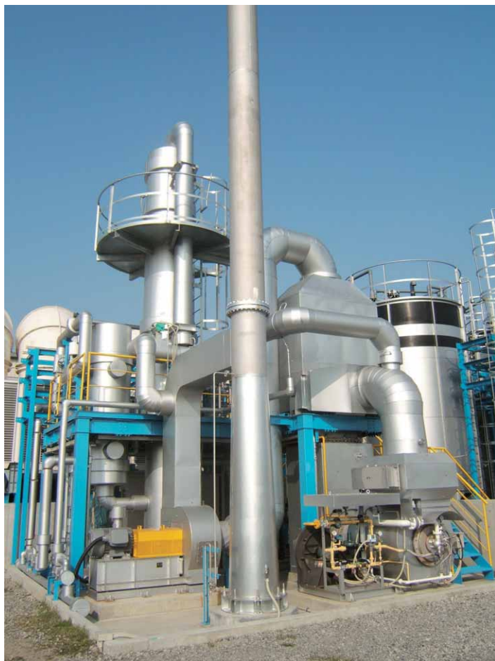
Ammonia gas decomposition system
