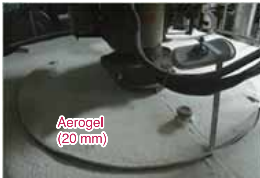
Upper part of boiler
