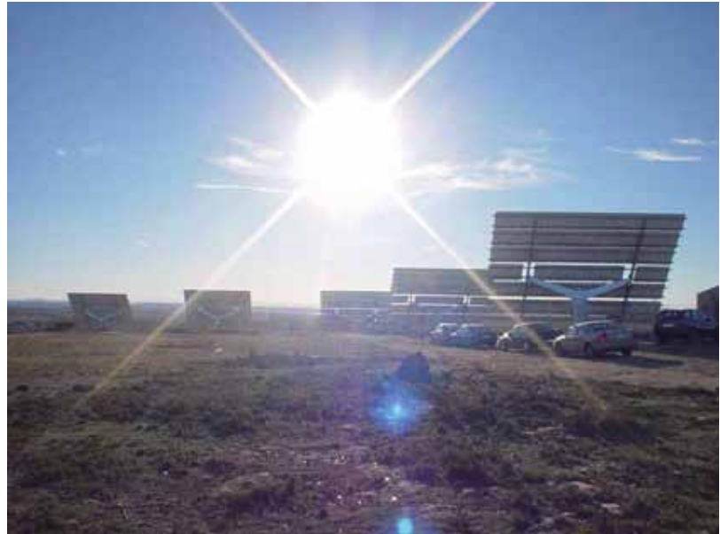
A Sun-tracking solar power system example
