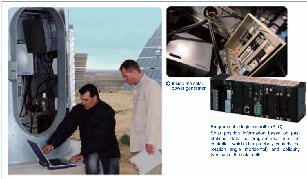
A Sun-tracking solar power system
