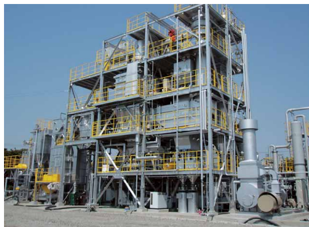
Plant proofing sewage sludge gasification and power generation
