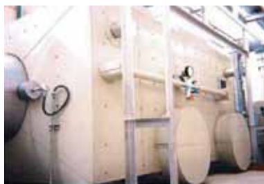
Appearance of Gas Denitrogenization Equipment (SCR Reactor)
