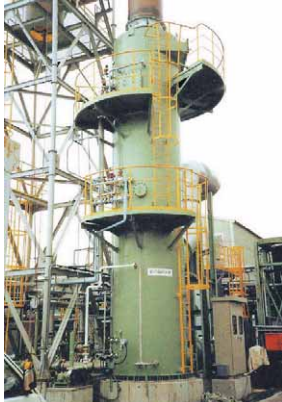
Appearance of Desulfurization Equipment
