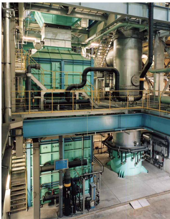
GREATS municipal waste incinerator hazardous gas elimination system
