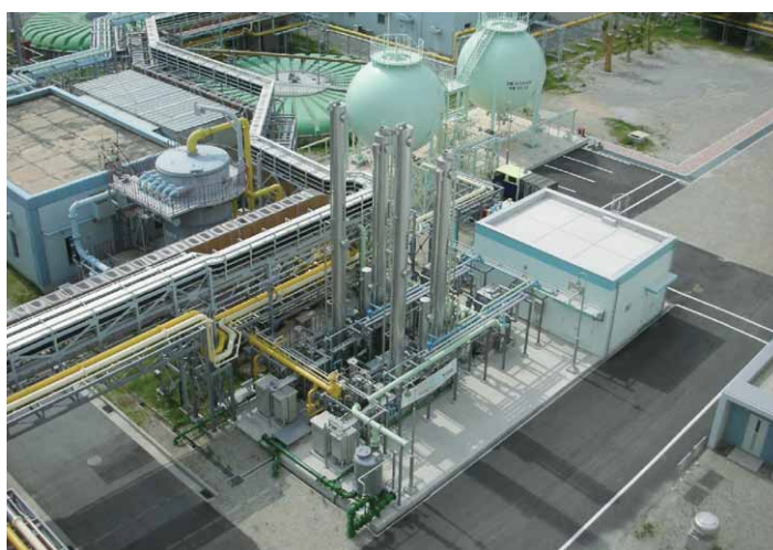
Refining equipment and gas tanks
