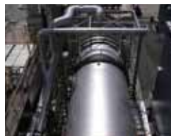
Heat treatment facility
